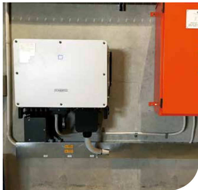
66kW PV Plant Prestons, NSW Australia 🇦🇺
